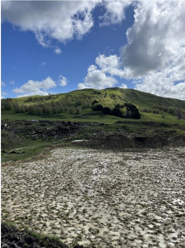
Figure 12: Looking west over extensive earthworks that have been carried out in the location of Lot 15. Source: Kate Hooper, 15 September 2022.
