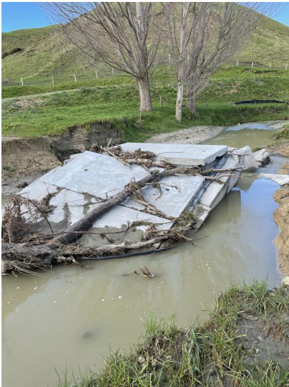
Figure 14: Damaged bridge preventing access to the other side of the stream where the beach access track is. Source: Kate Hooper, 15 September 2022.
