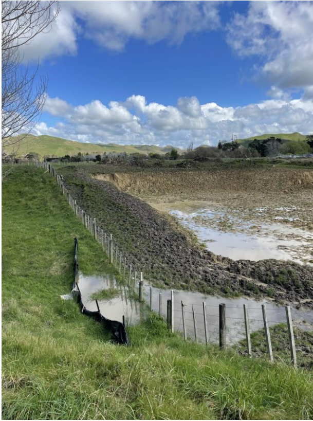
Figure 13: Looking south over extensive earthworks that have been carried out in the location of Lot 15. Source: Kate Hooper, 15 September 2022.
