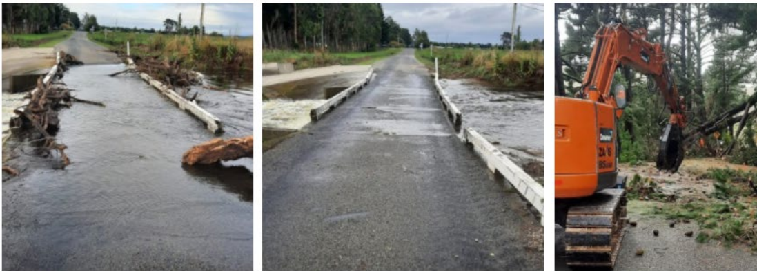
Herrick St, Taylors Slab Flooding. Before Photo
