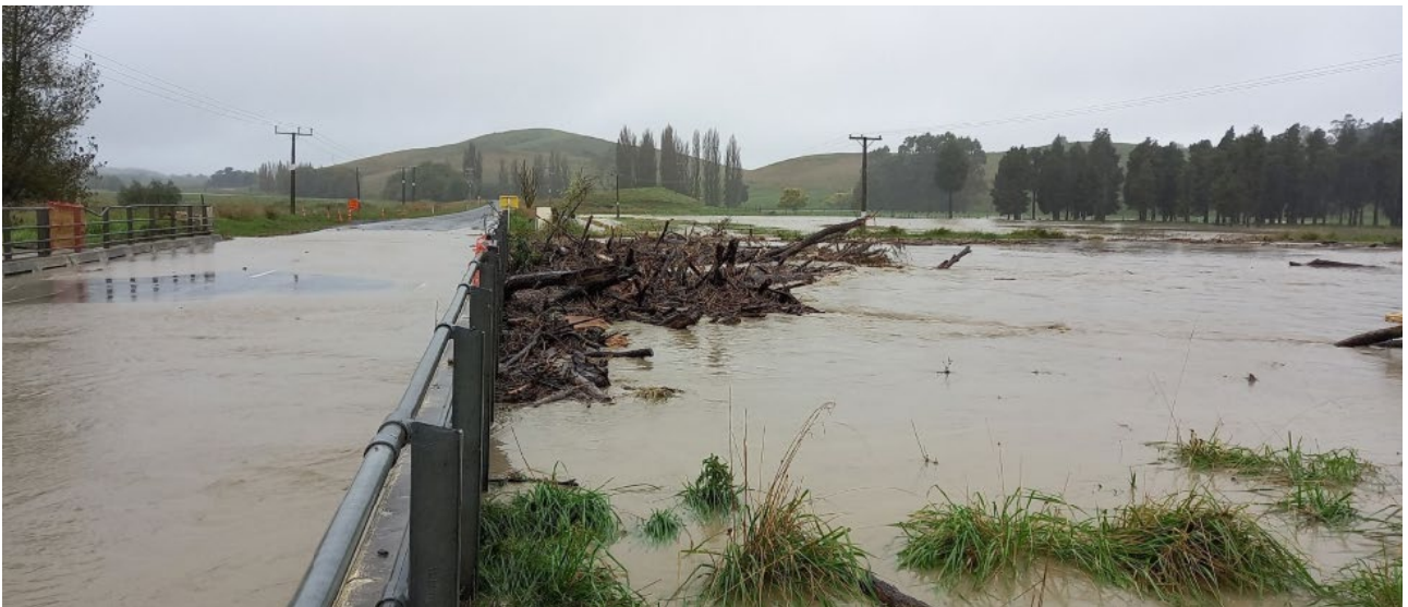
Figure 7: Flood waters and debris impacting Flaxmill Bridge – 24 th March 2022
