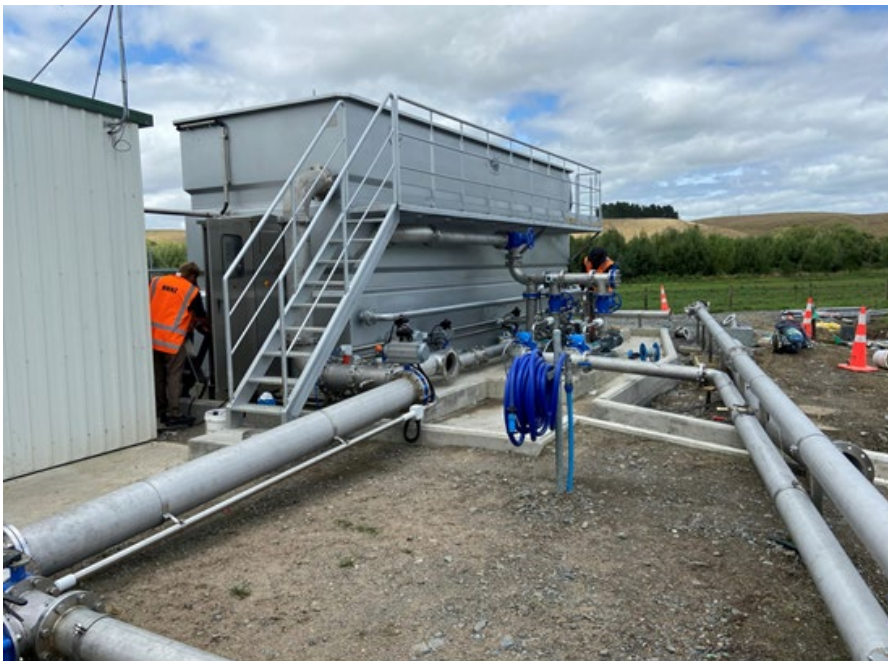
Figure 3: DAF in place
