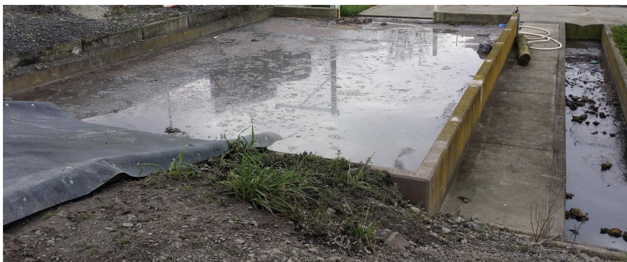
Figure 34: Waipukurau WwTP Concrete Drying Beds
