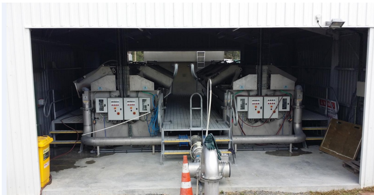
Figure 33: Waipukurau WwTP Sand Filter Building
