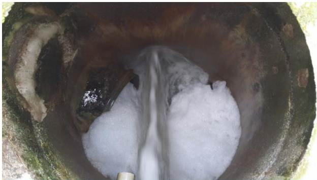
c) In the final effluent manhole
