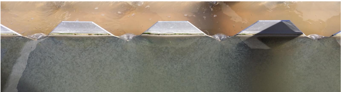
Figure 13: Solids Carry-Over from Lamella Tube Settlers at Waipukurau WwTP
