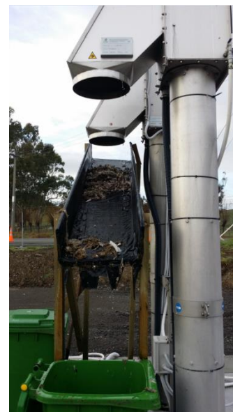
Figure 32: Waipukurau WwTP Inlet Screens
